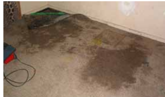
1. Prolonged leaking from shower making adjoining room unliveable
