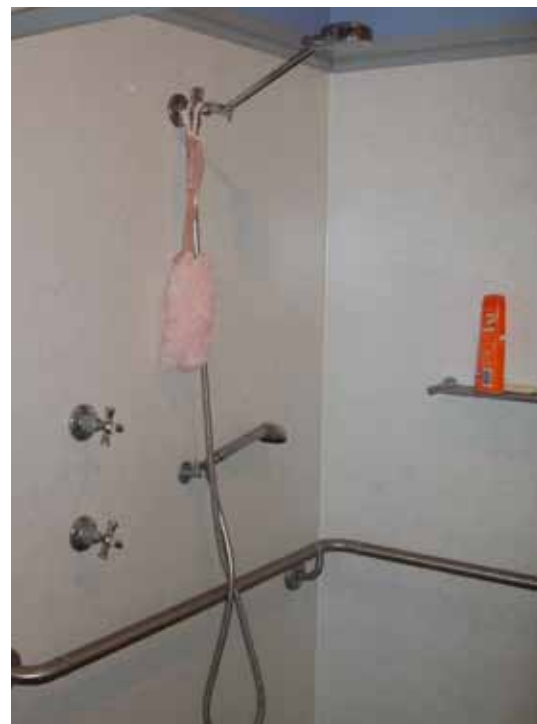
3. Completed shower rebuild. Where appropriate, advice is sought from local Occupational Therapists to ensure modifications suit the tenants' needs.
