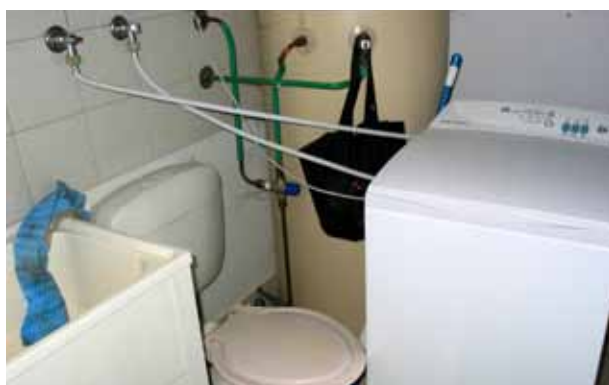
An example of poor original design of laundry plumbing
